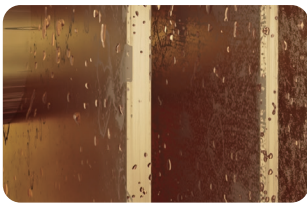
Water on Evaporator
